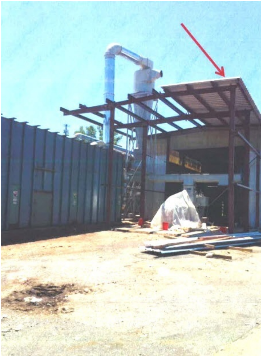
Northeast corner of the roof designated by the red arrow where the victim stepped off the roof falling approximately 24 feet.
